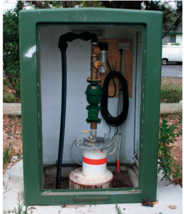
Groundwater Borefields Pump
