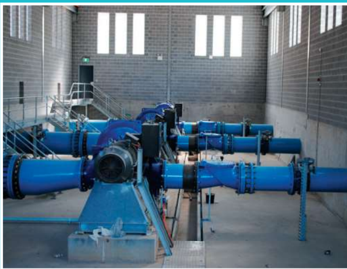
Mardi pumping station
